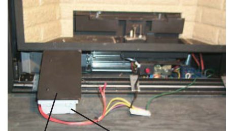
heat shield control box
