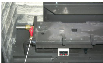
Shut off Valve
